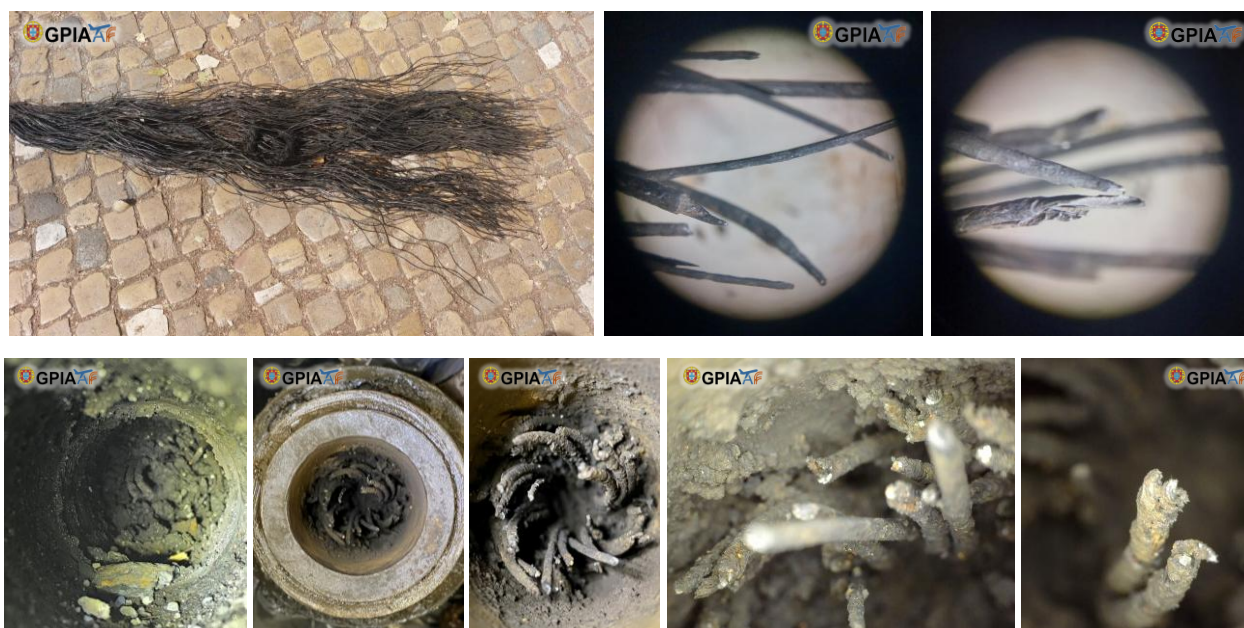
Fig. 12 - Close-up images of the wire fractures.
